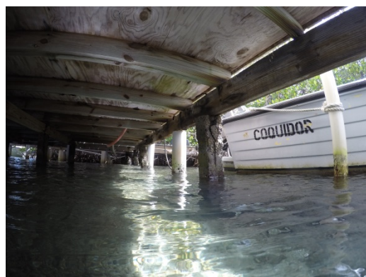
Northeastward View, under the diveshack Showing the deteriorated condition of cement pilings
