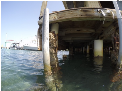
Northward View Showing deteriorated condition of cement piling
