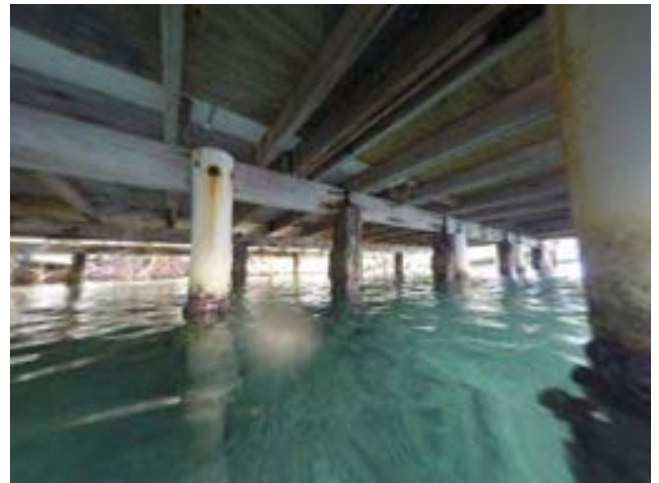
Diagonal View to the Southeast Showing the deteriorated condition of cement pilings
