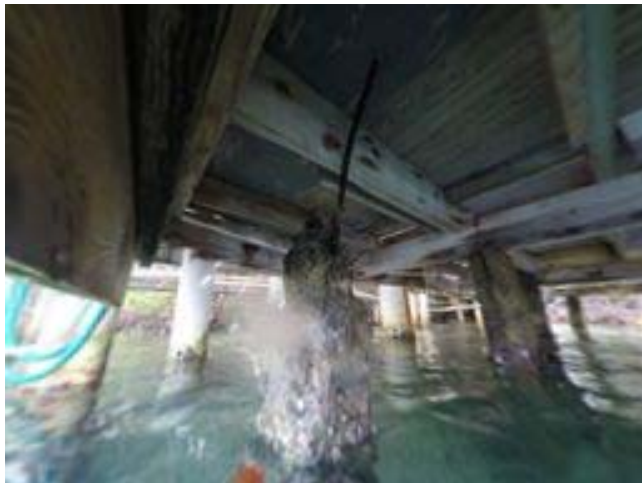
Diagonal View to the Northeast Showing the deteriorated condition of cement pilings
